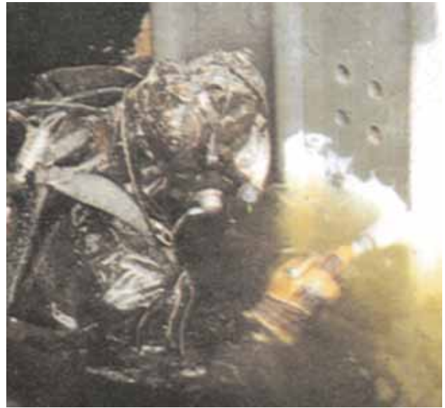
Above: A diver applies a second coat to a two-colour index system on sheet piling.
