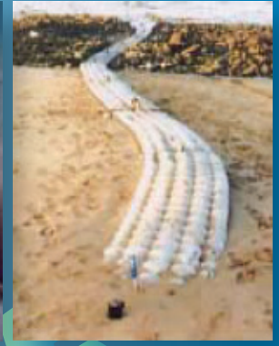
Protection mattress on small diameter pipeline.
